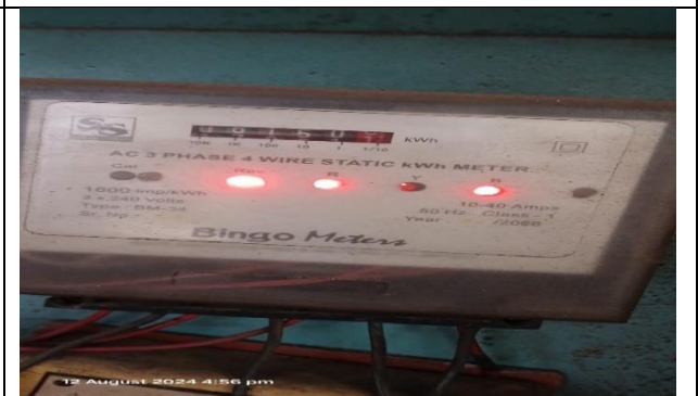
Photo 8: PETP energy meter
