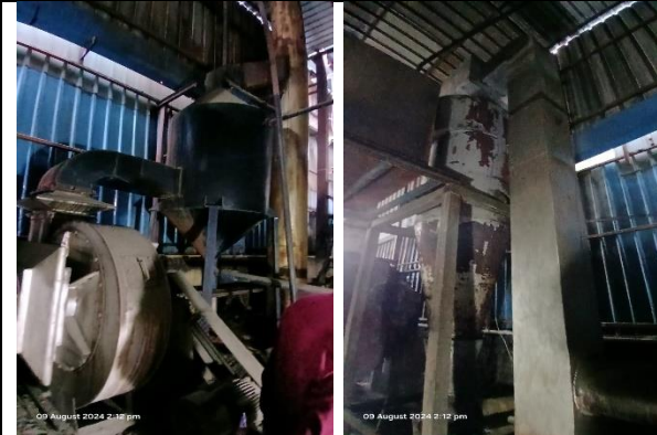
Photo 11: Air pollution control device
