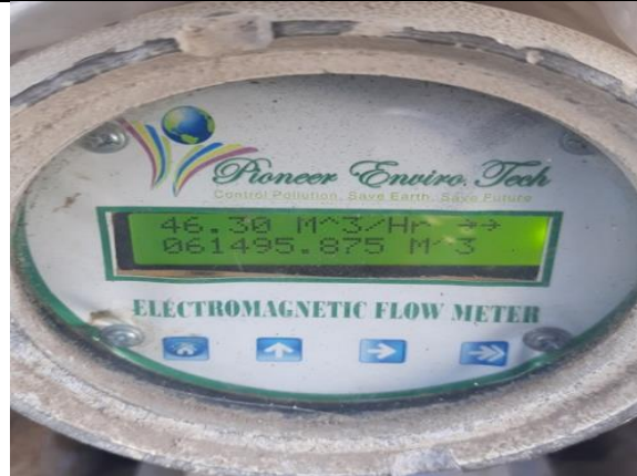
Flow meter installed at ETP Outlet
