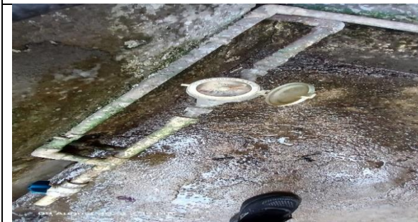
Photo 5: HSIIDC water supply line meter
