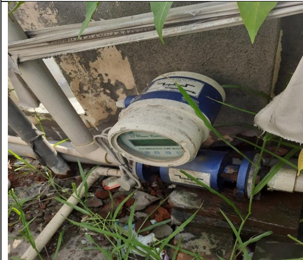
Flow meter (Defunct) installed at Borewell
