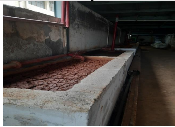
Sludge drying beds
