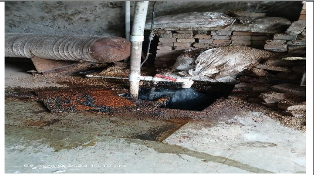
Photo 2: ETP inlet collection tank
