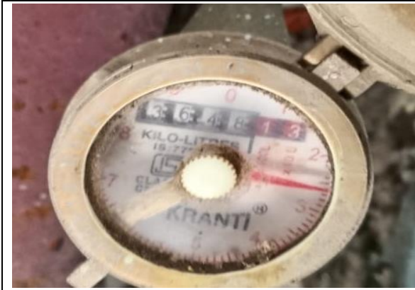
Flow meter installed at HSIIDC freshwater supply line
