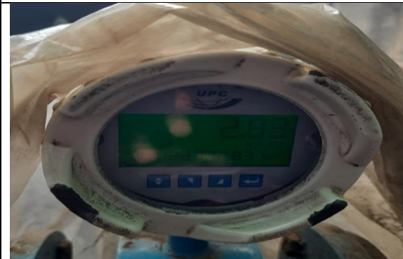
Flow meter installed at ETP Inlet
