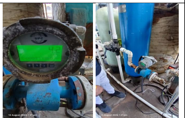
Photo 8: ETP outlet line with flow meter
