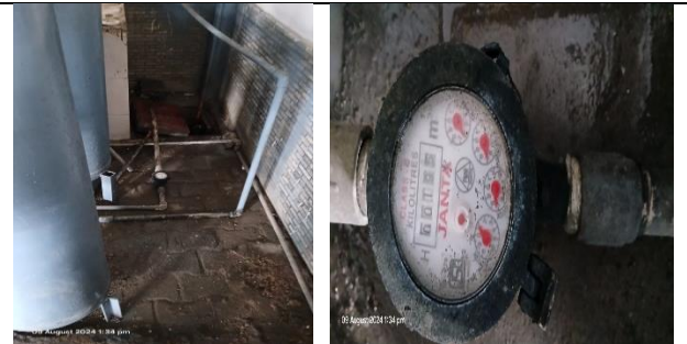
Photo 8: ETP outlet line with flow meter
