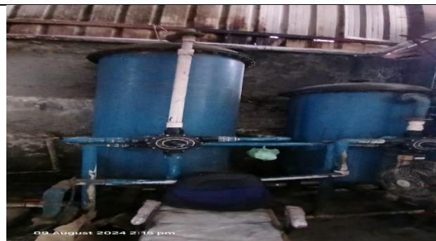
Photo 8: Tertiary treatment (Filtration) system
