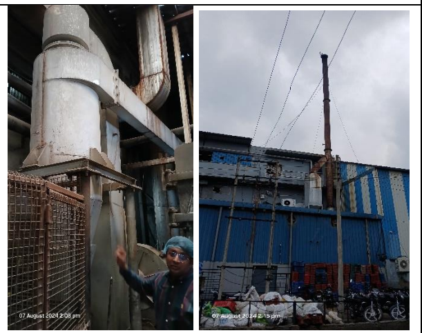
Photo 8: Air Pollution Control Equipment & Stack
