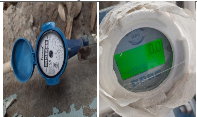
Flow meter installed at HSIIDC supply line & PETP Outlet
