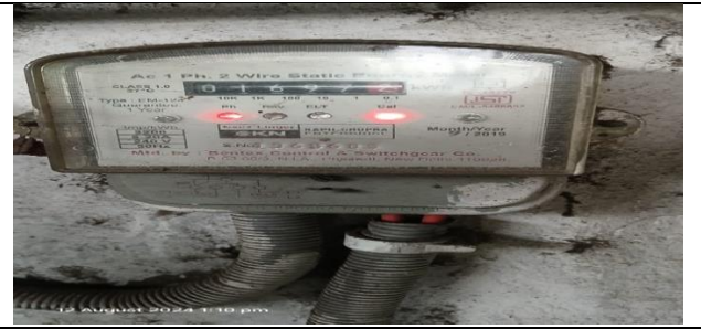
Photo 8: PETP energy meter
