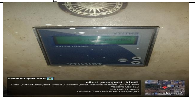
Fig.7: ETP energy meter
