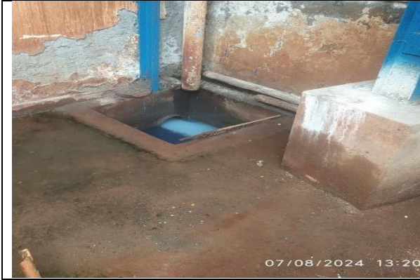
Fig.7: PETP unit (Tube Settler & settling tank) filled with clear water
