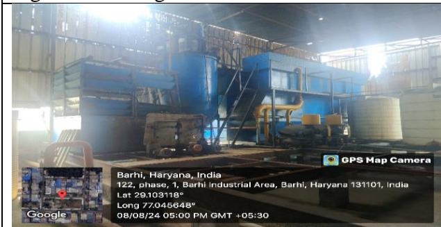
Fig.4: ETP set up
