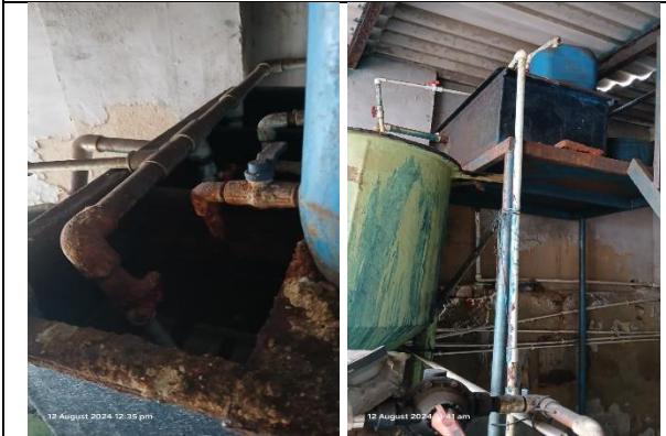
Photo 5: Chemical dosing system
