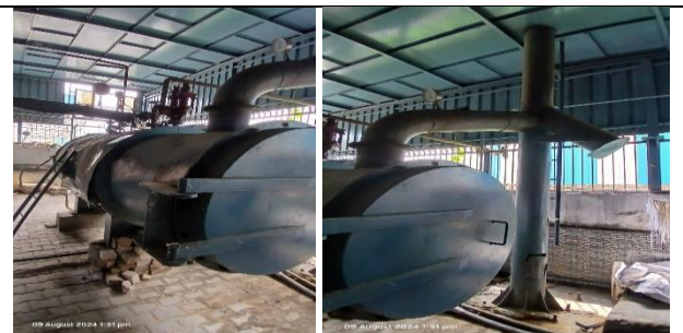
Photo 10: Boiler with stack
