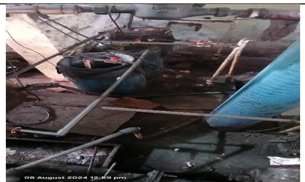
Photo 4: Chemical dosing system
