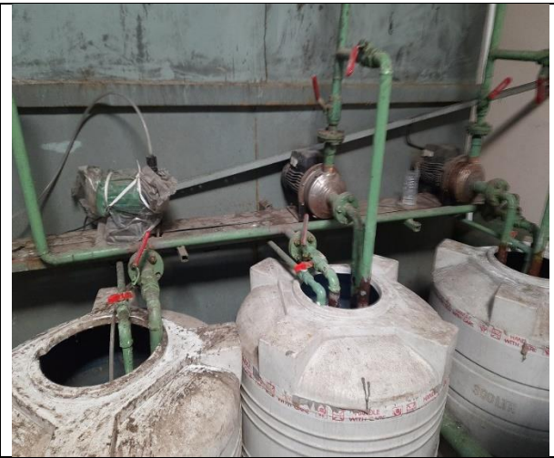
Chemical dosing at PETP
