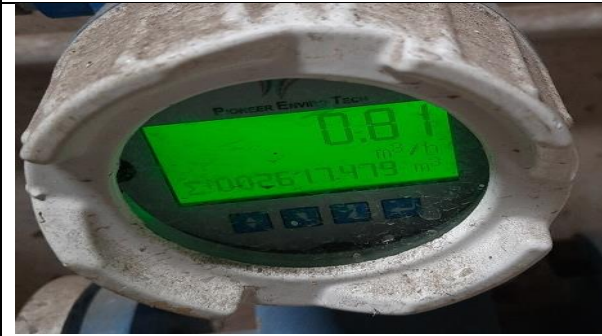
Flow meter installed at PETP Outlet
