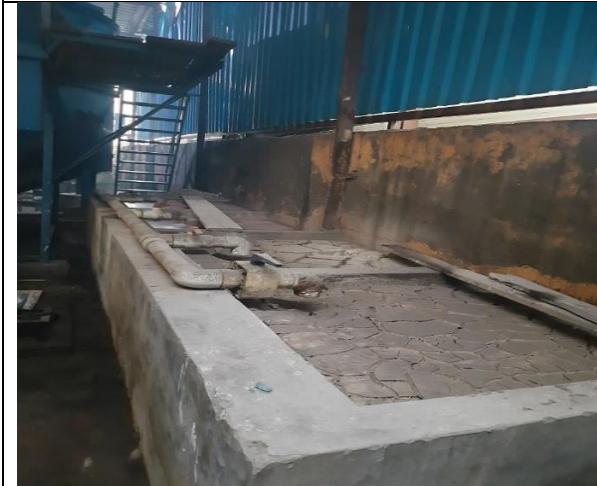
Sludge drying beds
