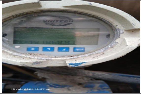
Photo 6: PETP outlet flow meter
