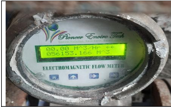
Flow meter installed at PETP Outlet
