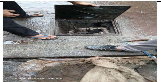
Photo 10: Borewell without flow meter
