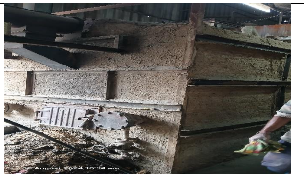
Photo 6: Boiler with stack
