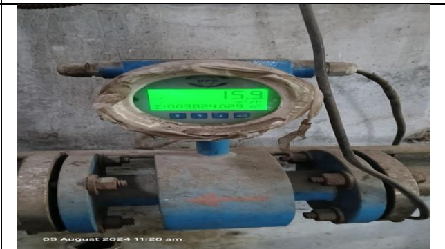
Photo 4: ETP Inlet flow meter
