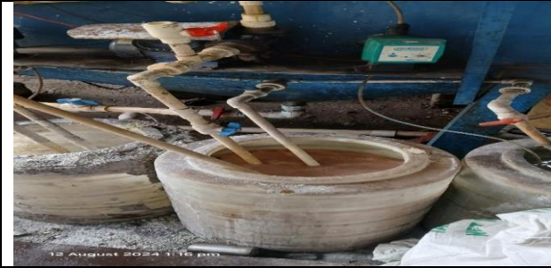
Photo 5: Chemical dosing system
