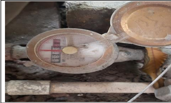
Flow meter installed at HSIIDC freshwater line
