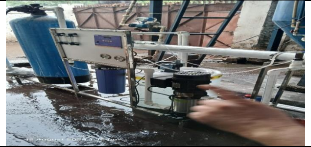
Photo 6: RO system in PETP
