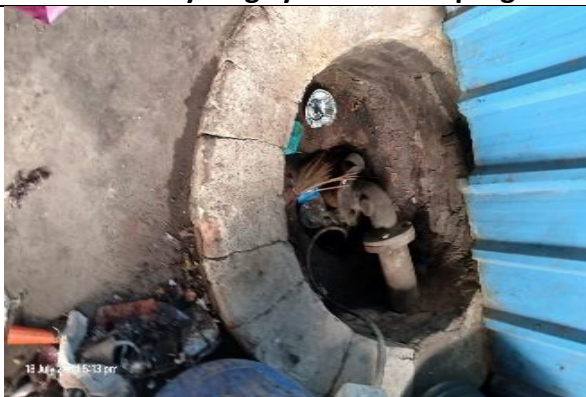
Photo 13: Borewell without flow meter
