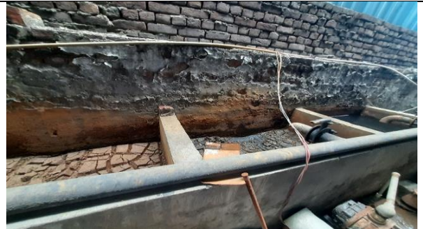
Sludge drying beds
