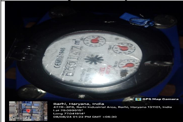
Fig.6: PETP inlet flow meter
