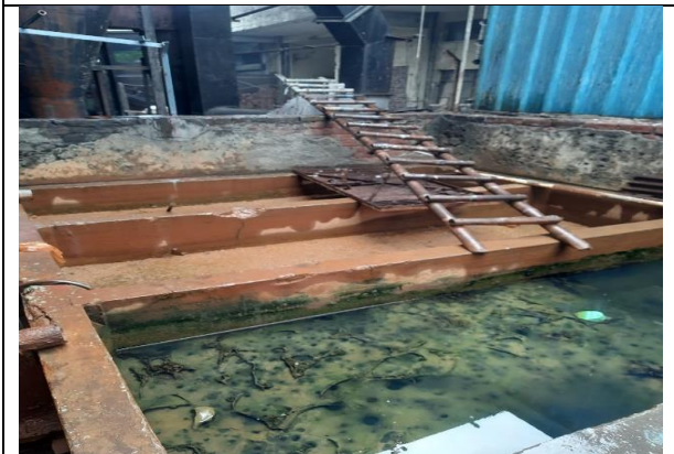
Sludge drying bed
