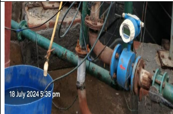
Photo 10: PETP outlet flow meter
