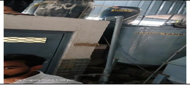
Photo 4: Chemical dosing and reaction tank
