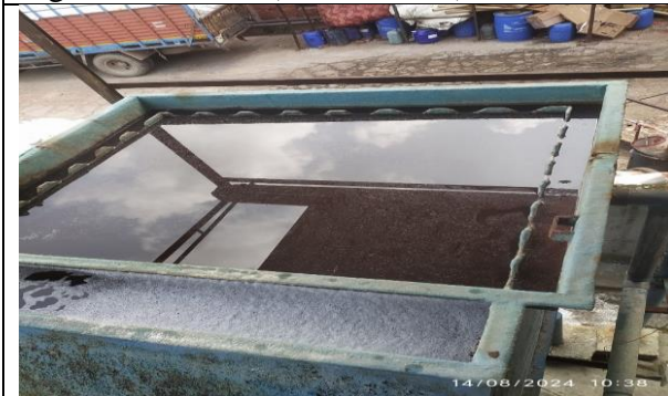
Fig.9: PETP inlet flow meter
