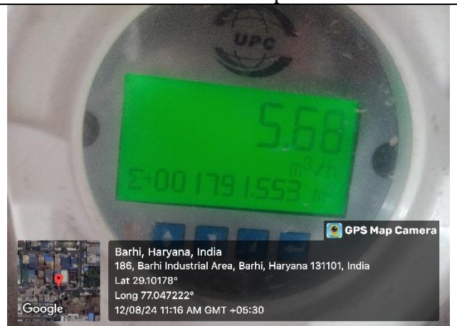
PETP inlet flow meter
