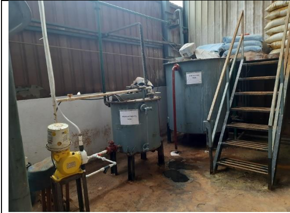
Chemical dosing at ETP
