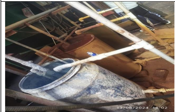
Fig.11: Sludge drying beds
