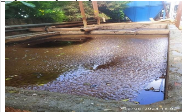
Fig.13: PETP Inlet & outlet
