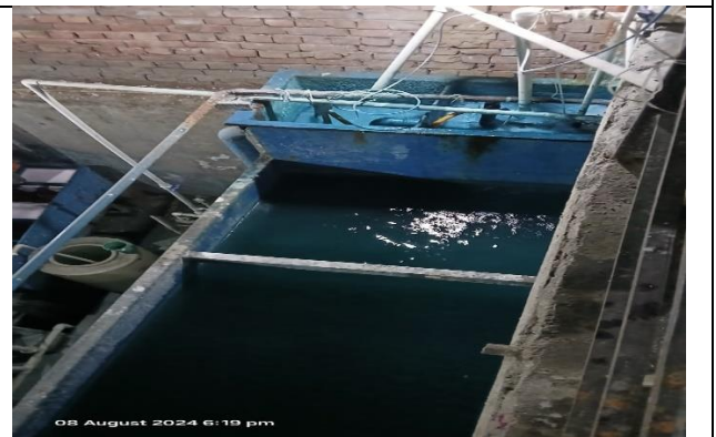
Photo 6: Chemical reaction tank & tube settler
