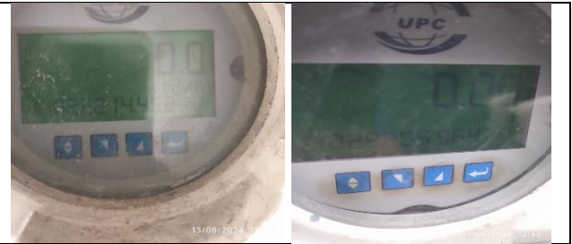
Fig.8: PETP energy meter
