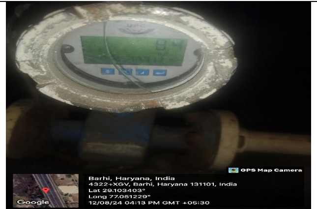
PETP outlet flow meter
