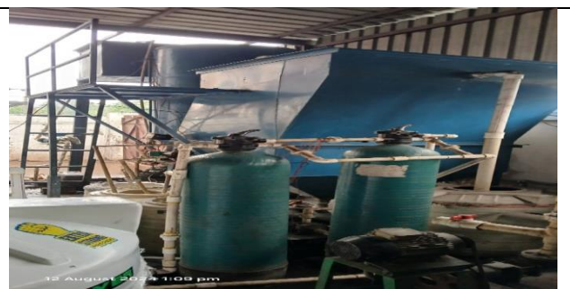
Photo 4: Chemical reaction tank, tube settler & filtration units
