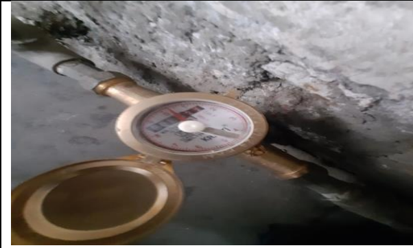
Flow meter installed at HSIIDC freshwater line-2
