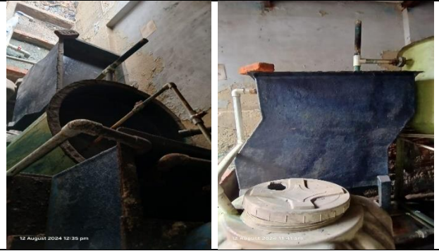
Photo 4: Chemical reaction tank & tube settler
