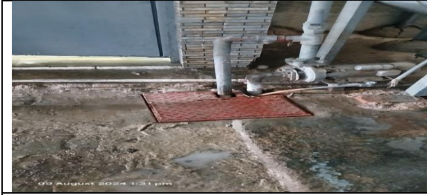
Photo 3: PETP inlet collection tank
