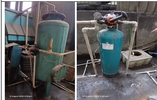
Photo 5: Carbon filter and Resin filter
