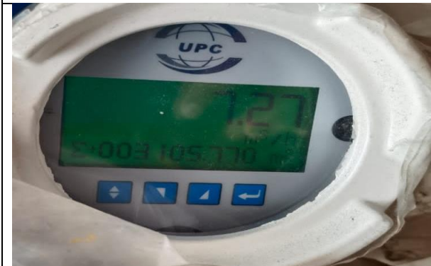
Flow meter installed at PETP inlet
