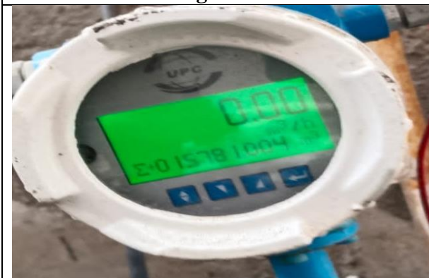
Flow meter installed at Borewell
