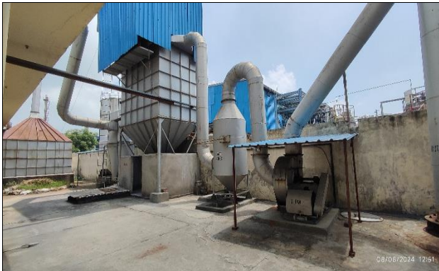
Photo 1: Cyclone and wet scrubber
