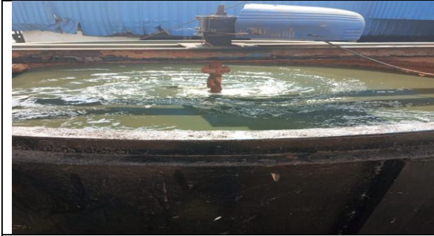
Fig.9: PETP unit (tube settler) & Aeration tank cum settling tank with diffused aeration with media
