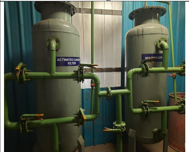
Activated Carbon Filter & Multigrade Filter
