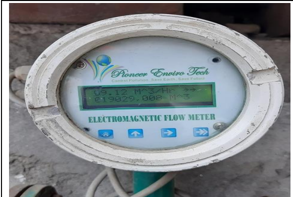
Flow meter installed at PETP Outlet
