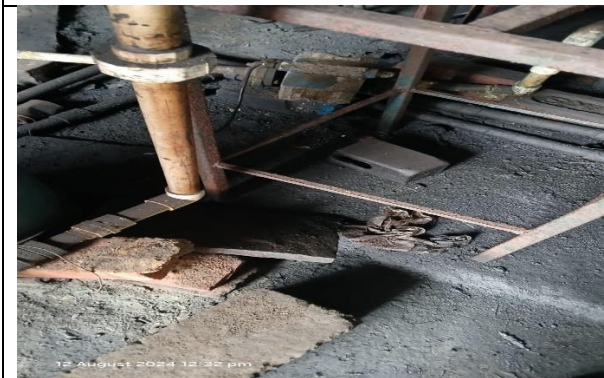
Photo 9: PETP inlet flow meter
