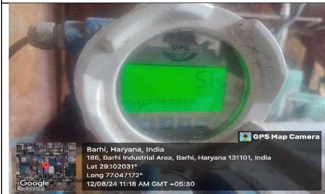
PETP outlet flow meter
