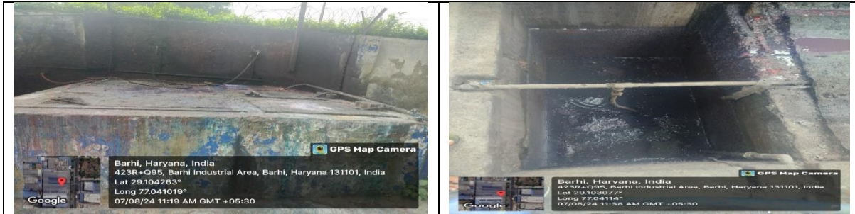
Screen washing area
