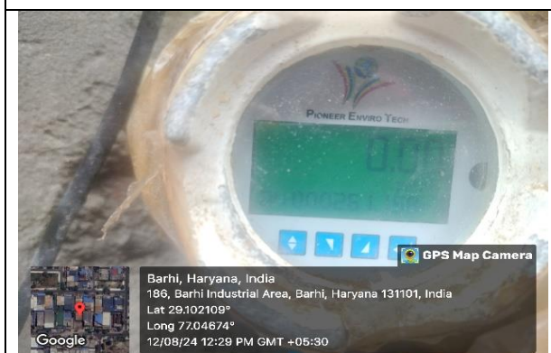
Fig.3: PETP inlet flowmeter
