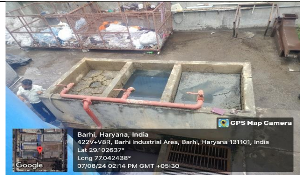
Fig.9: Sludge Drying Beds
