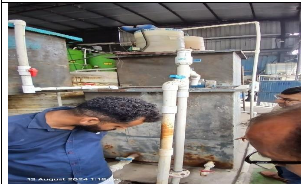
Photo 5: Overall ETP system
