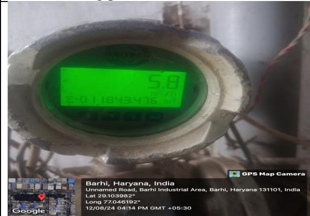
PETP inlet flow meter
