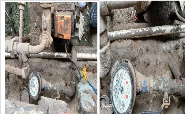
Photo 7: HSIIDC water line flow meter
