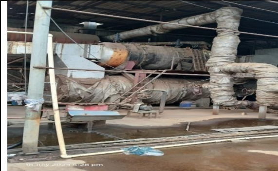
Photo 8: Thermopack for steam generation
