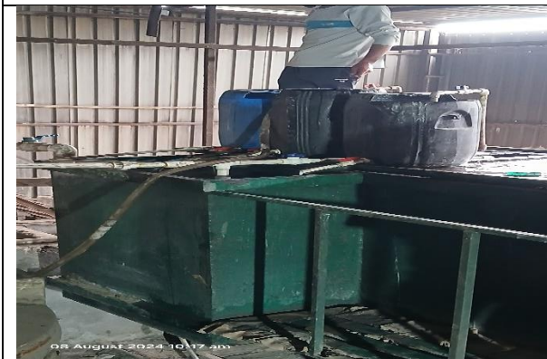
Photo 3: Chemical dosing and reaction tank
