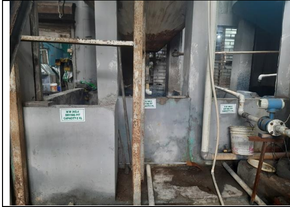
Sludge drying beds
