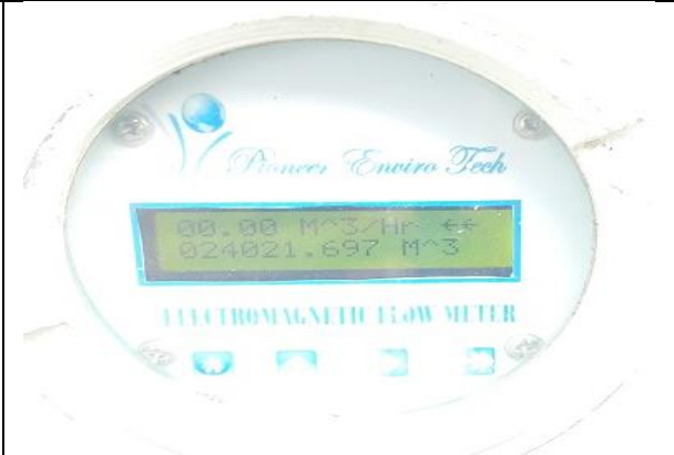
Flow meter installed at PETP Outlet
