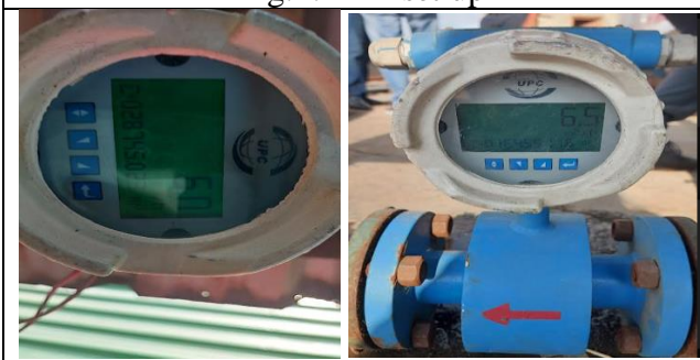
Fig.6: ETP inlet & outlet flow meter
