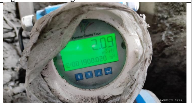
Fig.6: ETP outlet flow meter
