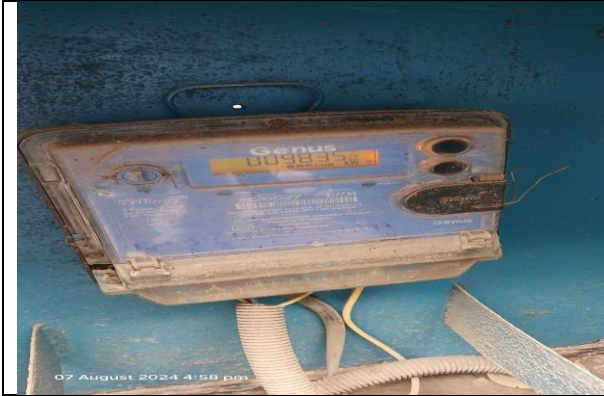
Photo 7: PETP energy meter
