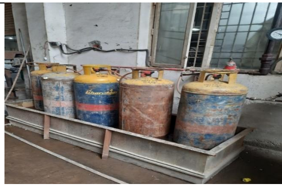
Fuel (LPG) used in Boiler
