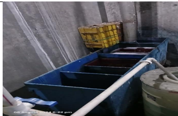
Photo 5: ETP inlet bar screen
