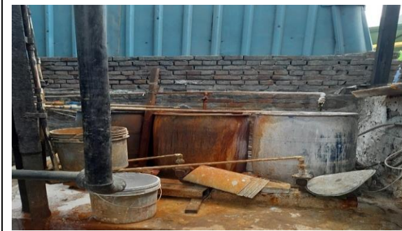
Chemical dosing at PETP
