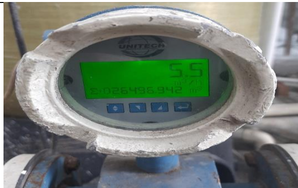
Flow meter installed at PETP Inlet
