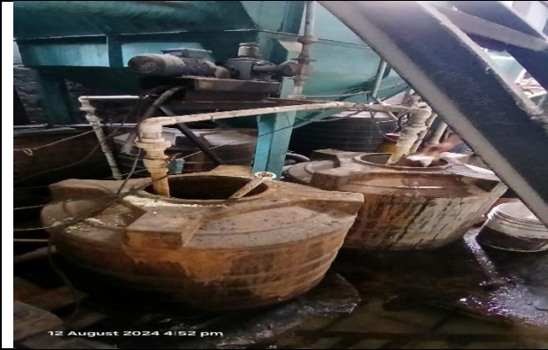
Photo 9: Chemical dosing system
