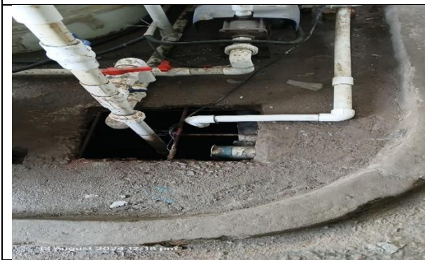
Photo 3: ETP inlet collection tank
