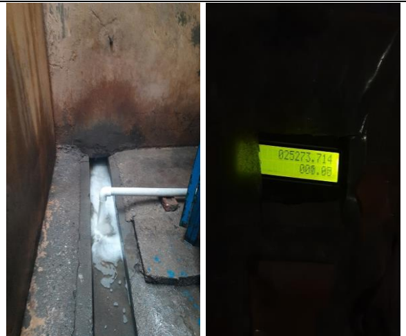
PETP Outlet & Flow meter
