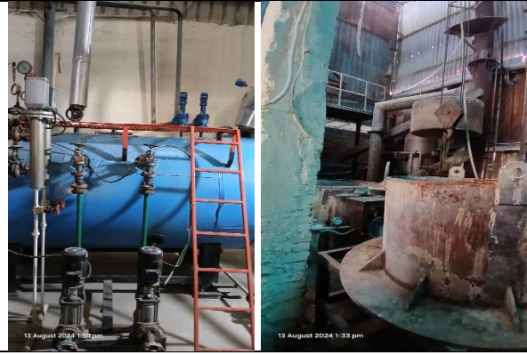
Photo 10: Boiler & wet scrubber with stack
