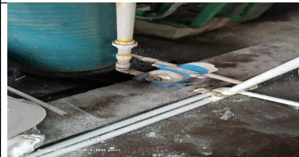
Photo 9: PETP inlet flow meter
