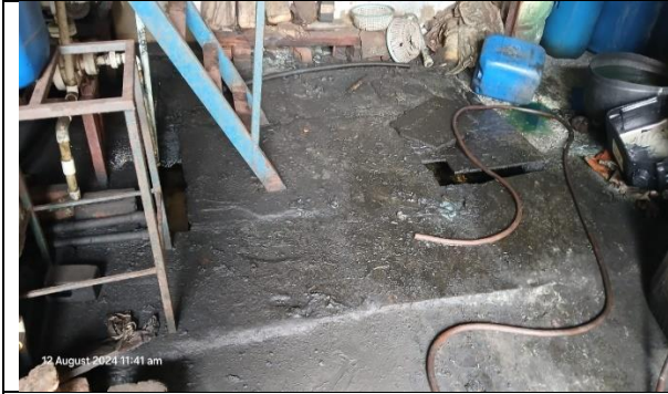
Photo 3: PETP inlet collection tank
