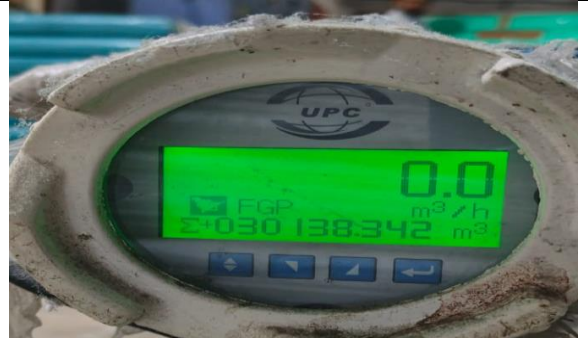
Flow meter installed at Borewell
