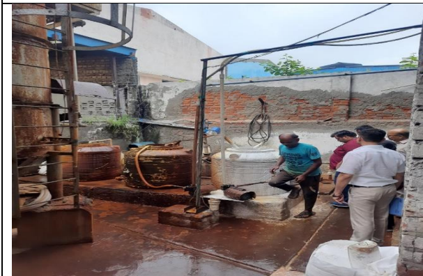
Chemical dosing at PETP
