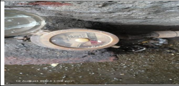
Photo 7: HSIIDC water line flow meter
