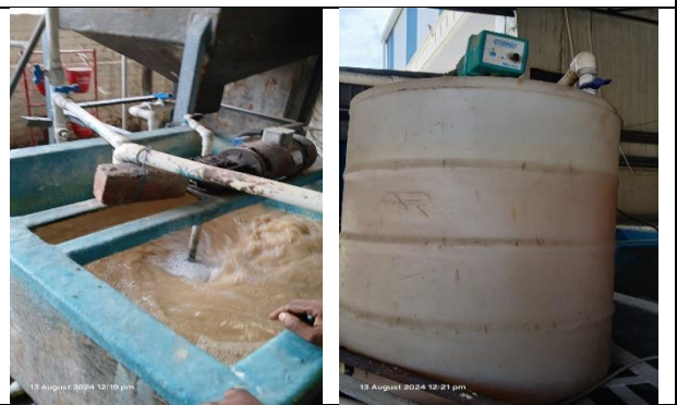
Photo 4: Chemical dosing and reaction tank
