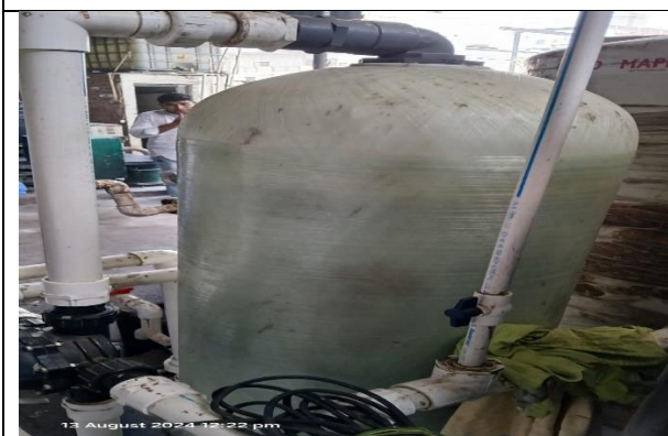
Photo 7: Softener at ETP outlet
