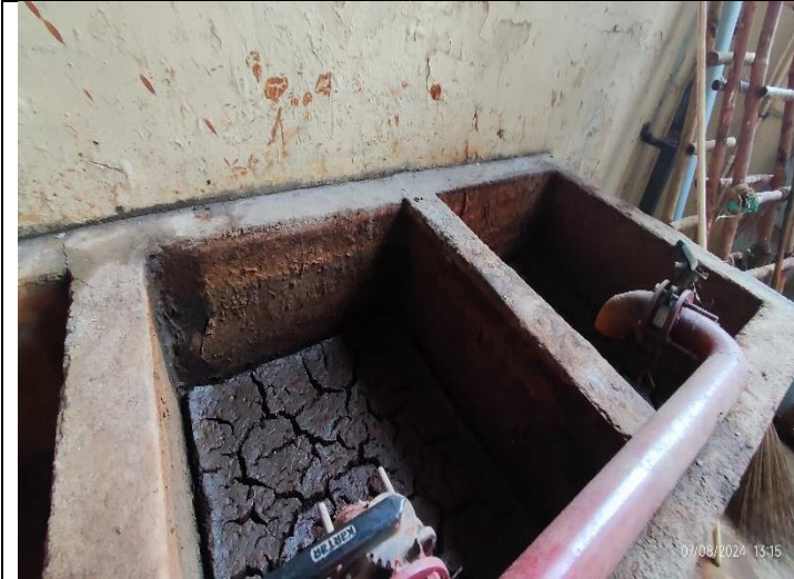
Fig.5: Sludge drying bed
