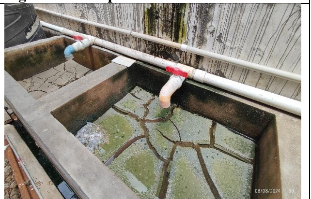
Fig.8: Sludge drying bed
