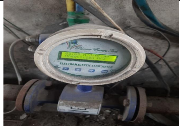
Flow meter installed at PETP Outlet
