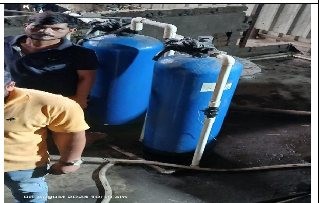
Photo 4: Filtration units in ETP
