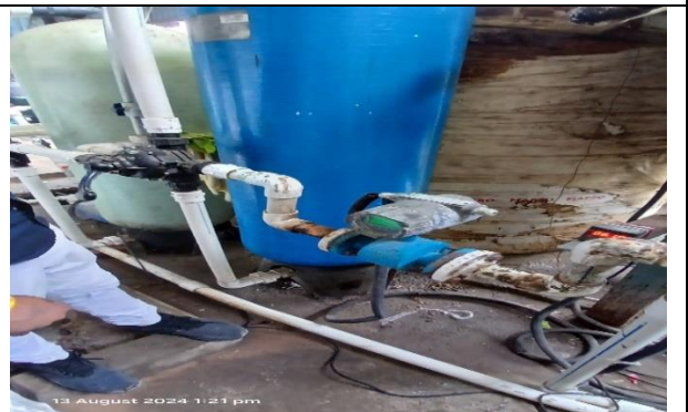
Photo 6: Filtration units in ETP
