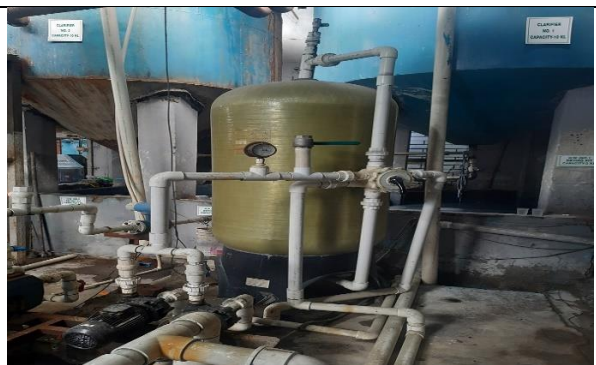
Clarifiers & Media filter
