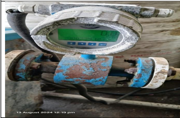
Photo 11: ETP inlet flow meter
