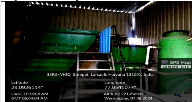
Fig.7: PETP inlet flow meter
