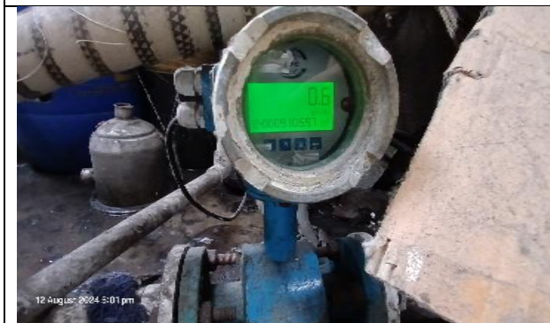
Photo 7: PETP outlet flow meter
