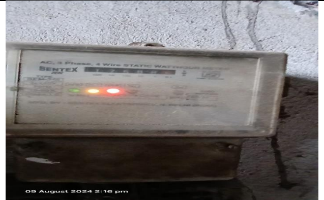
Photo 12: Energy meter at ETP
