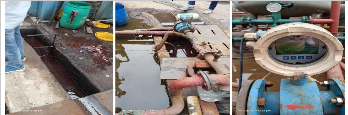
Photo 3: PETP Inlet channel with screen, collection tank and inlet flow meter
