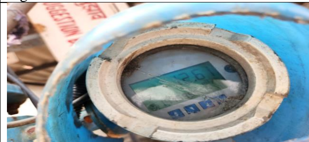
Fig.10: Flow meter reading of Borewell-2
