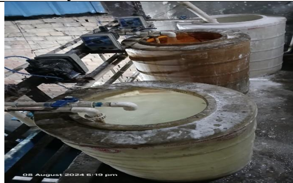
Photo 9: Chemical dosing system (mechanical)
