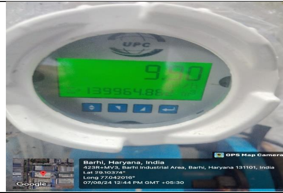
PETP Outlet flowmeter
