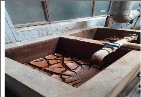
Sludge drying beds
