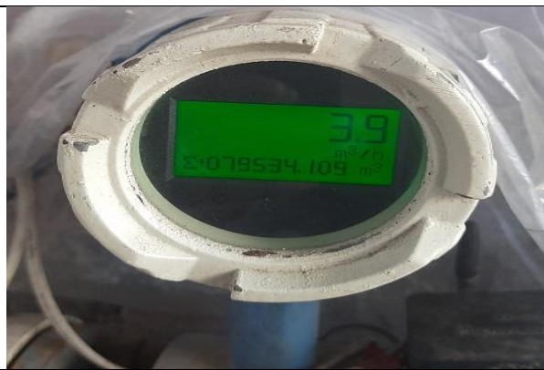
Flow meter installed at Bore-well
