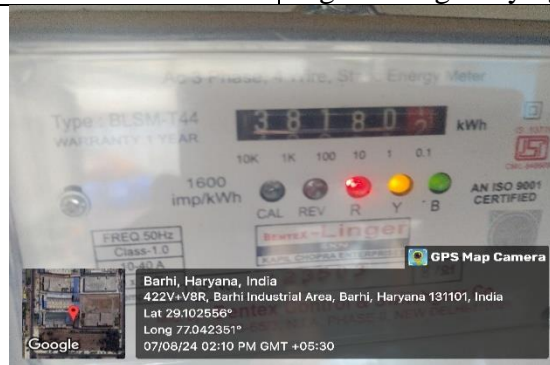
Fig.10: PETP energy meter
