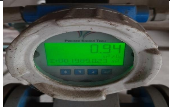
Flow meter installed at PETP Inlet
