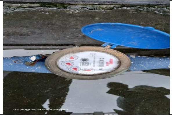
Photo 8: PETP outlet flow meter
