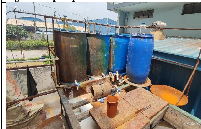
Fig.7: ETP flash mixer tank (with tap)
