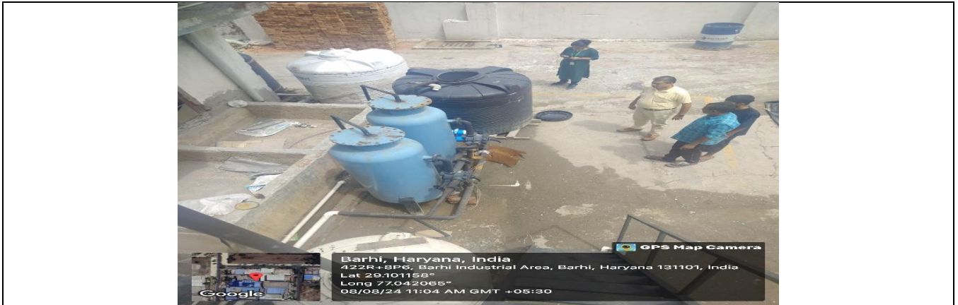
Sludge drying bed and Treated water tank (Black in colour)
