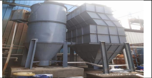
Fig.8: Boiler and wet scrubber
