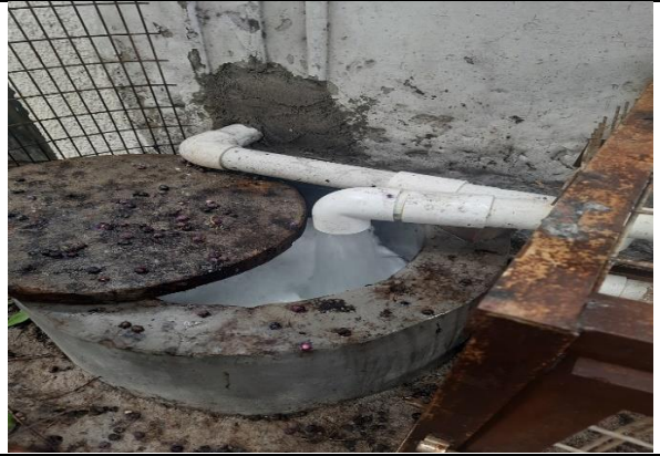
Treated effluent disposal point
