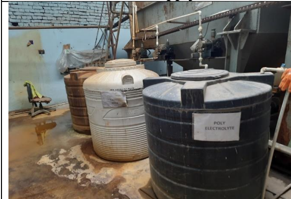
Chemical dosing at PETP
