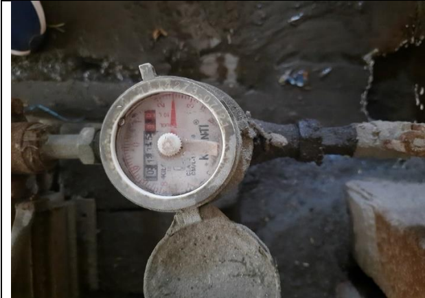
Flow meter installed at HSIIDC supply line
