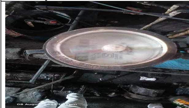
Photo 7: ETP outlet flow meter
