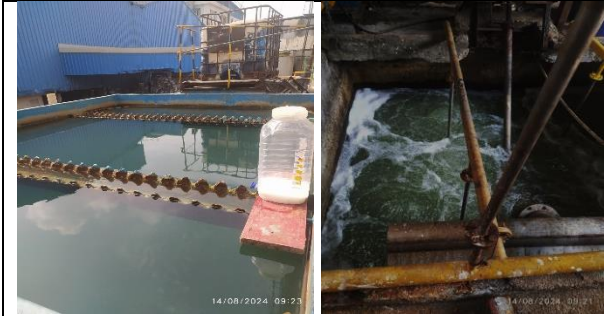
Fig.11: PETP unit (Press filter) & Sludge storage
