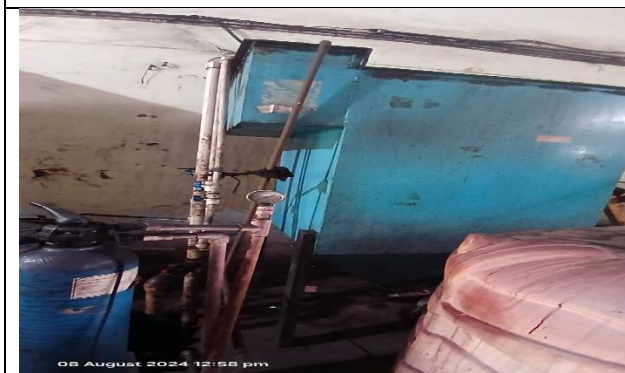
Photo 3: Chemical reaction tank & tube settler
