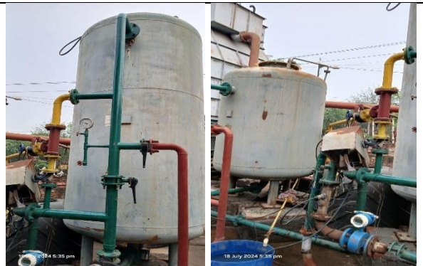
Photo 5: Tertiary treatment (Resin column)
