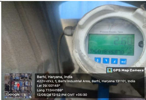
PETP outlet flow meter
