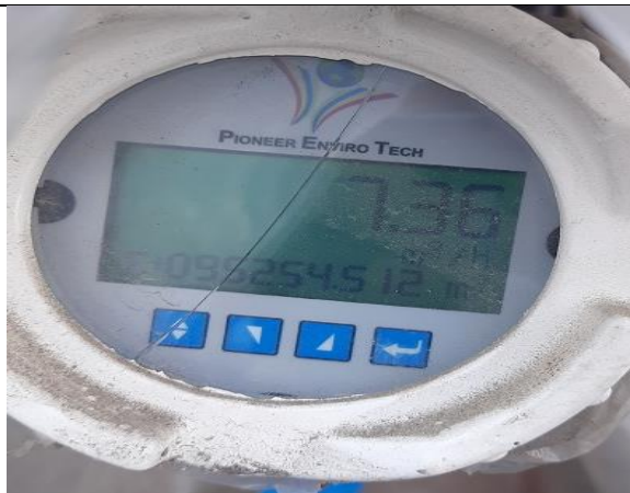
Flow meter installed at Borewell
