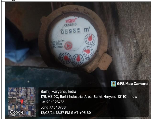
Fig.7: HSIIDC water flow meter
