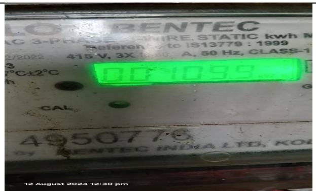
Photo 10: PETP energy meter
