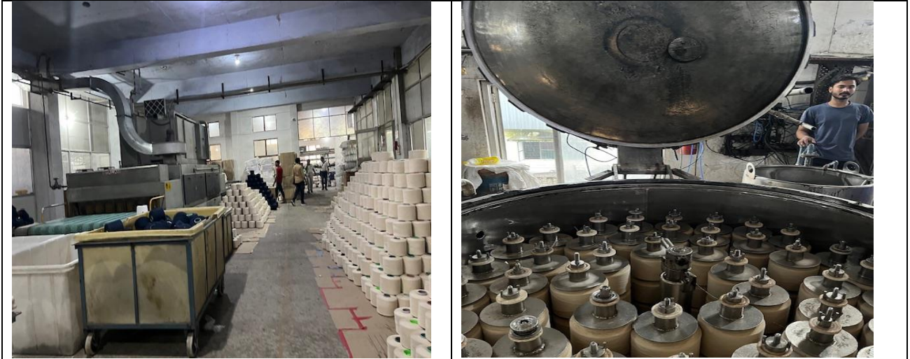
Fig.3: PETP - chemical dosing & Tube settler
