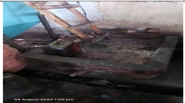
Photo 8: Sludge drying beds found empty
