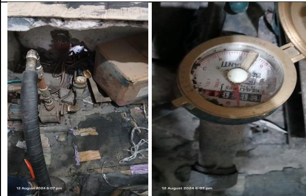
Photo 11: HSIIDC water supply line with flow meter
