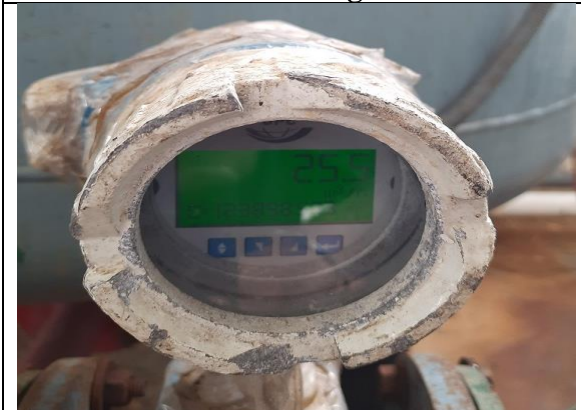
Flow meter installed at ETP Inlet
