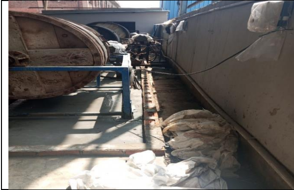
Fig.5: Underground wastewater collection pit cum Equalization Tank
