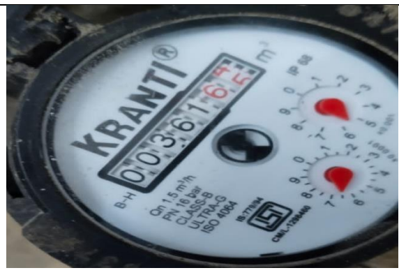
Flow meter installed at HSIIDC supply
