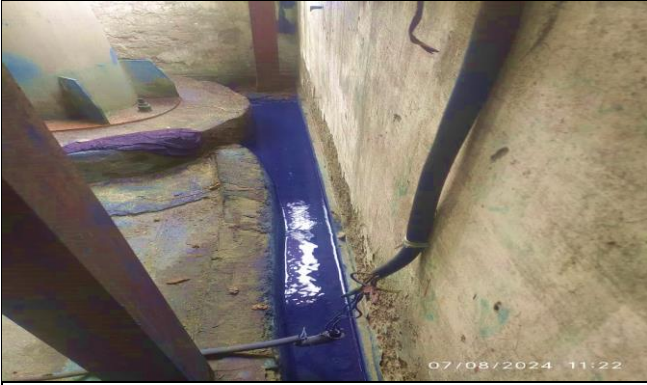
Photo 11: PETP outlet Flowmeter (disconnected wire)
