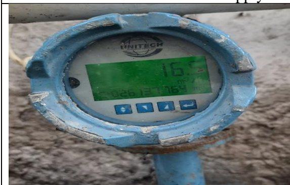
Flow meter installed at PETP Outlet
