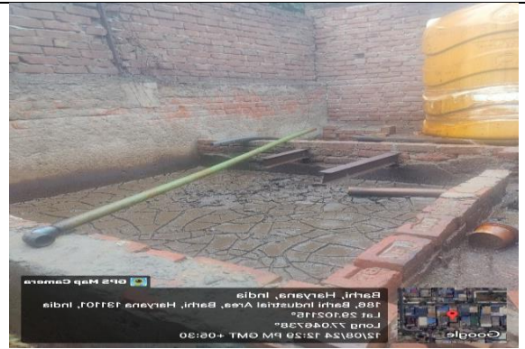
Fig.6: Sludge drying bed
