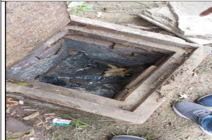
PETP outlet discharge point
