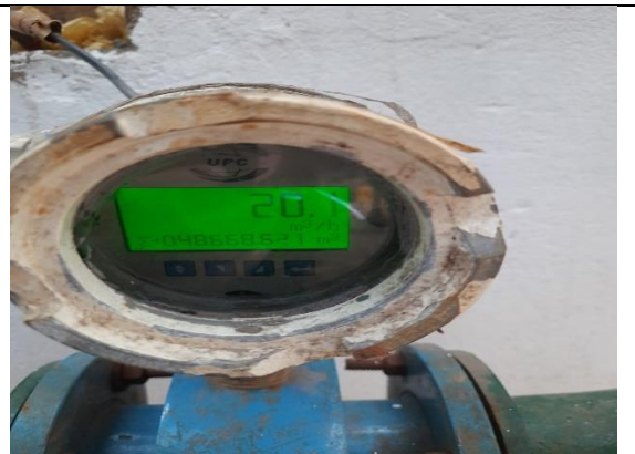
Flow meter installed at ETP Inlet
