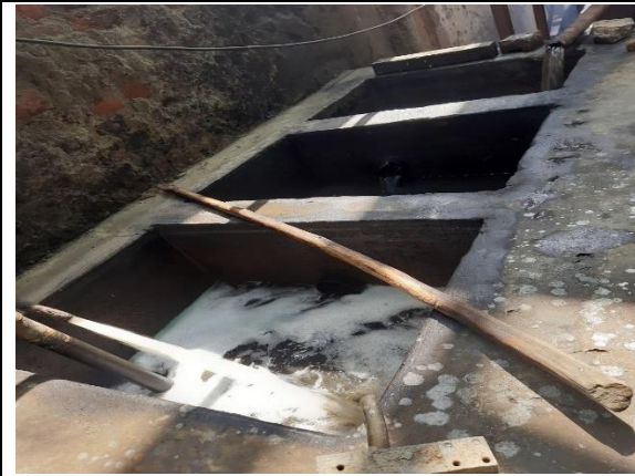
Sludge drying beds
