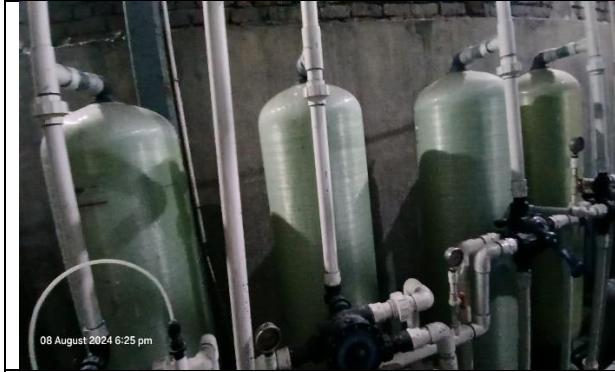
Photo 7: Tertiary treatment (Filtration) system
