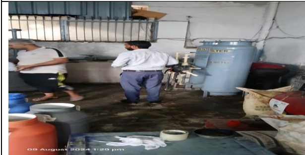
Photo 7: Filtration units in PETP
