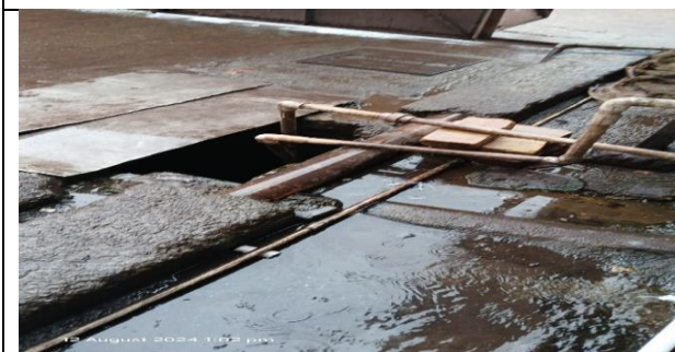
Photo 3: PETP inlet collection tank
