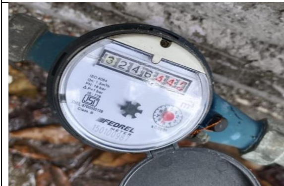
Flow meter installed at HSIIDC supply line
