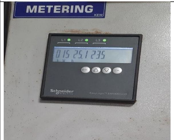
Energy meter installed at PETP
