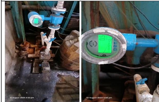
Photo 3: PETP inlet line flow meter
