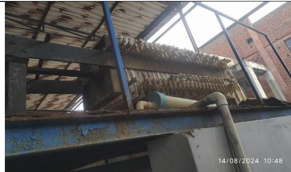
Fig.8: PETP unit (Chemical mixing tank)
