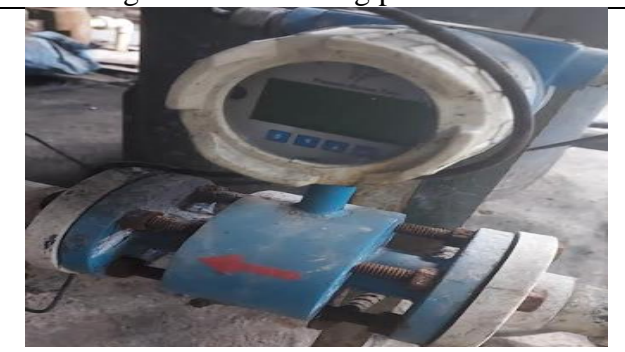
Fig.4: PETP inlet flow meter
