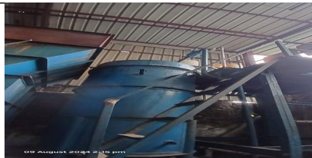
Photo 6: Chemical reaction tank
