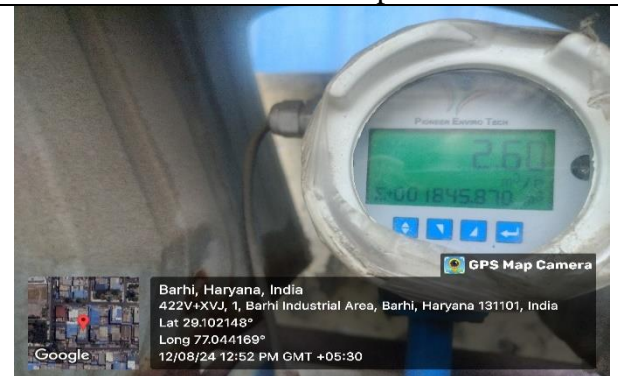
PETP inlet flow meter
