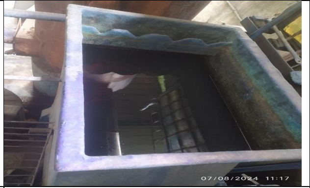
Photo 12: Sludge Dewatering unit (Filter press)
