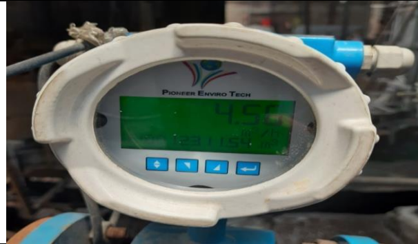
Flow meter installed at PETP Inlet
