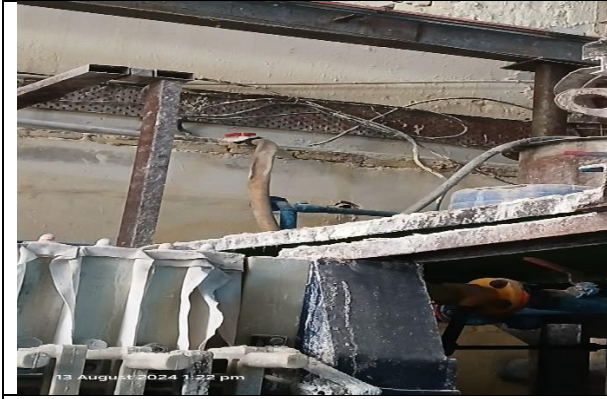
Photo 9: Treated effluent reuse location
