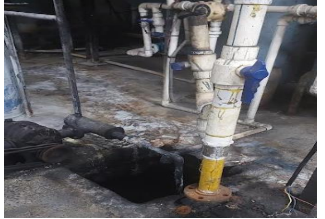
Fig 6. Outlet Motor before filters sent to repairing
