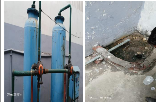
Photo 9: PETP Tertiary filtration units & outlet
