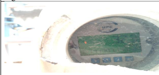
Fig.9: Flow meter reading of Borewell-1
