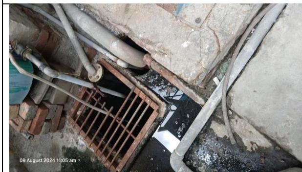
Photo 5: ETP inlet collection tank
