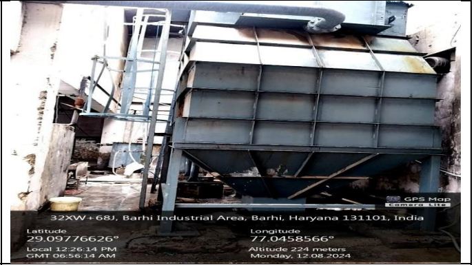
Fig.6: ETP outlet flow meter
