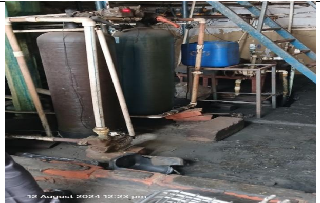
Photo 6: Tertiary treatment (Filtration) system
